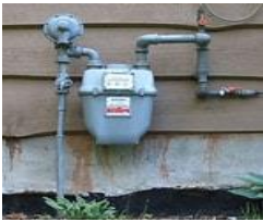
Natural gas meter
